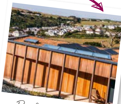
Roof solar panels
